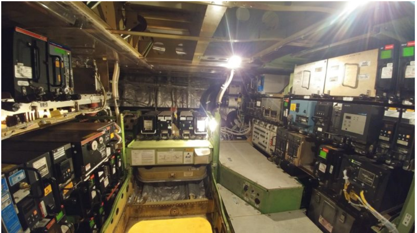
The avionics bay
